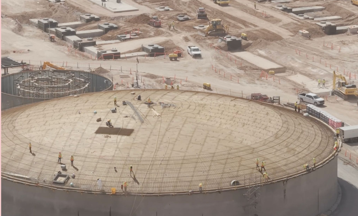
A water tank at the Meta Data Center site in El Paso.
