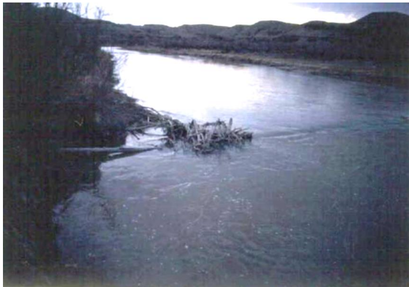
Examples of exposed pipeline (Fogg and Hadley, 2007 from Hydroquest report)
